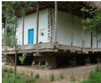
Figure 6. Walls are not connected to the ground so are protected from moisture
