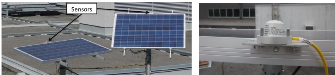
Fig.2: Picture showing details on the mounting of the pyranometers (left) on the two PV panels, and (right) close-up of the sensor support
